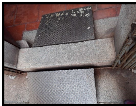
Figure 2 The additional ramp provided as facilities passage for the person with disabilities. (Source: Author, 2026)
