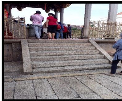
Photo 1: There are no facilities such as ramps and a hand holder provided for senior citizens and disabled people to visit the heritage building.
