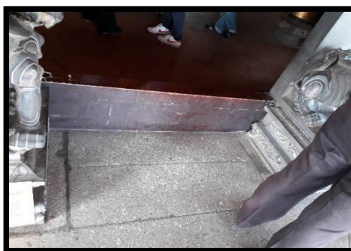
Photo 3: The high sill that prevented the wheelchair to get to the other side of the building.
